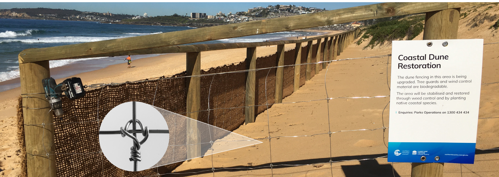
Strong Lock installed at Northern Beaches, NSW with magnified view of the superior lock joint
